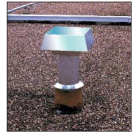
roof mounted hood
